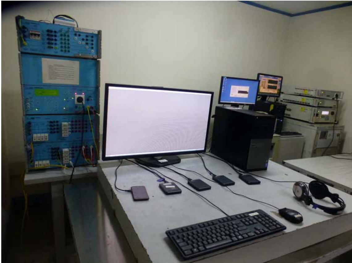
15.7. Photo of Surge Test
